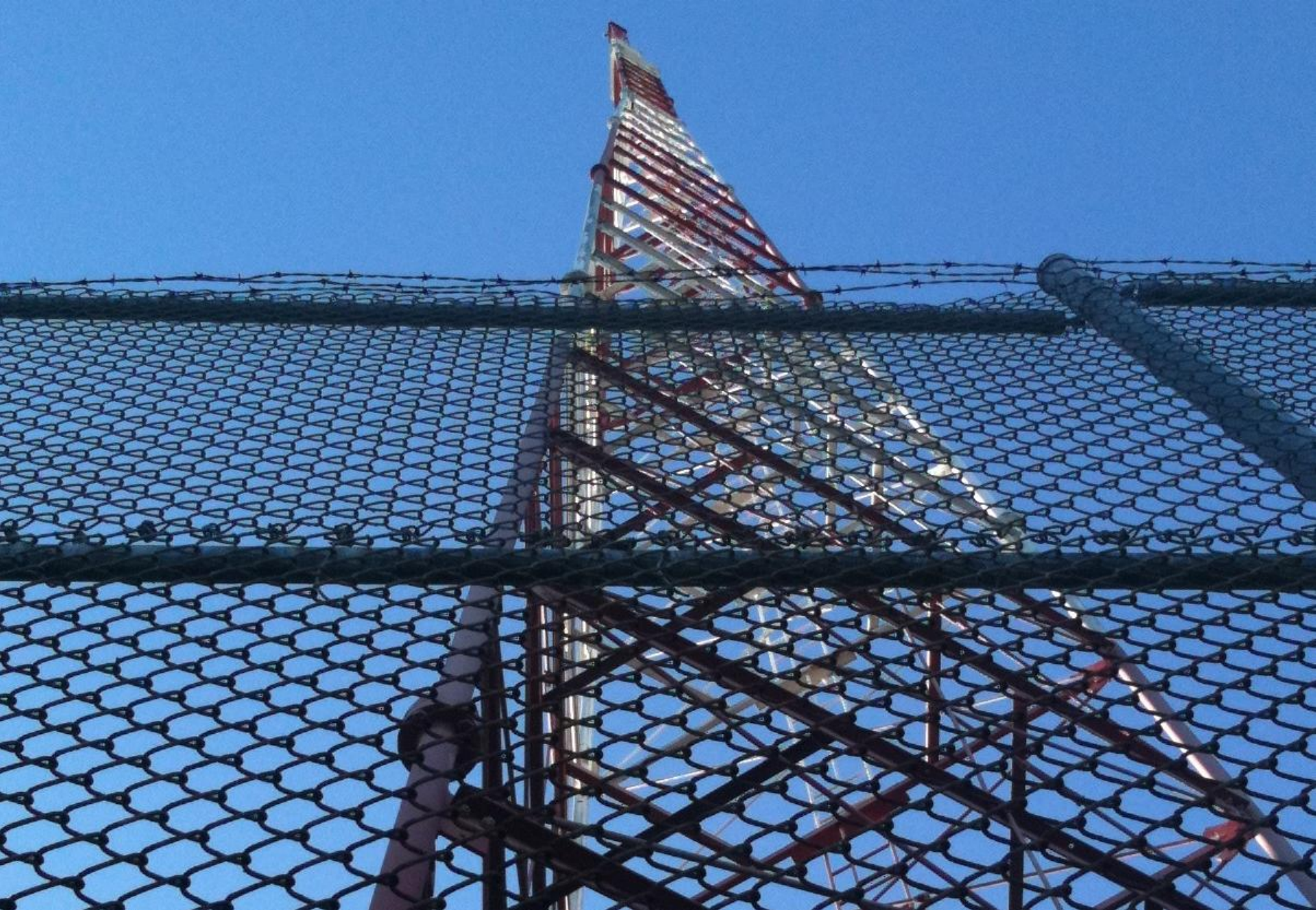
Grounding At Commercial Radio Station KESE Monterey – 1.2 MHz (1240)
